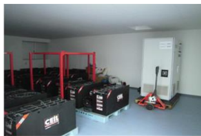
30 fork trucks batteries & Power control unit
