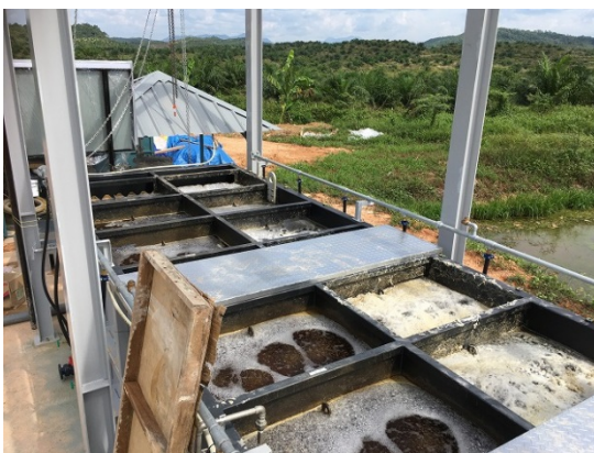
Wastewater Treatment System (April 2018)
