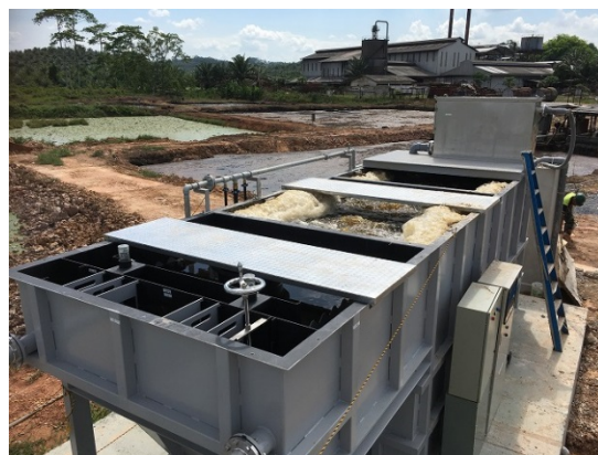
Wastewater Treatment System (April 2018)
