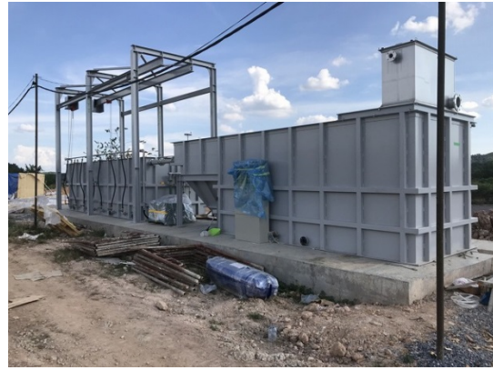
Installed Wastewater Treatment System (March 2018)
