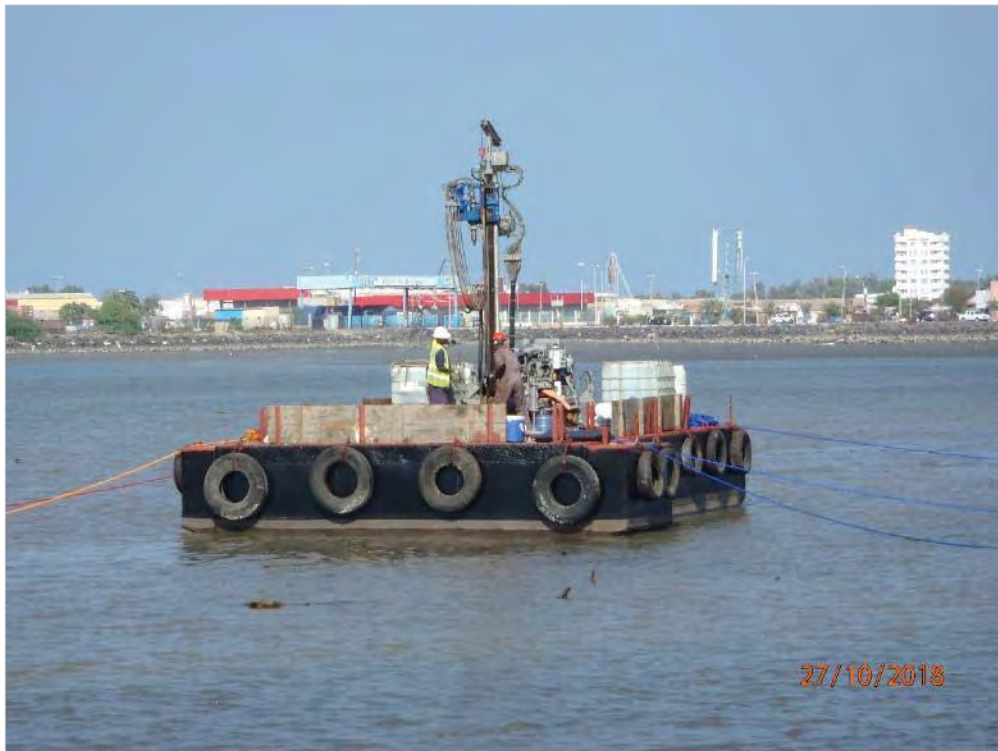
Photography 1: Floating pontoon
