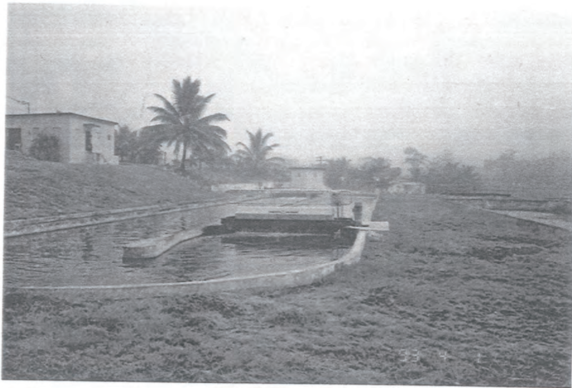
Plate 15 Charlemont Housing Scheme Sewage Treatment Plant.
