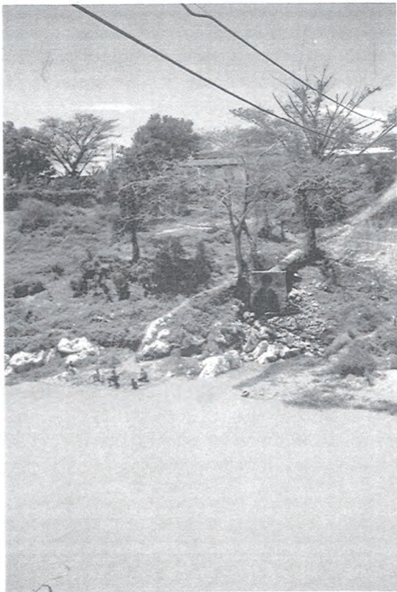
Plate 21 - Culvert taking wastewater into Rio Cobre in Spanish Town.
