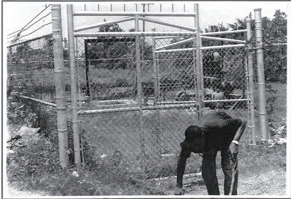
Plate 3 - Duhaney Park lift station.
