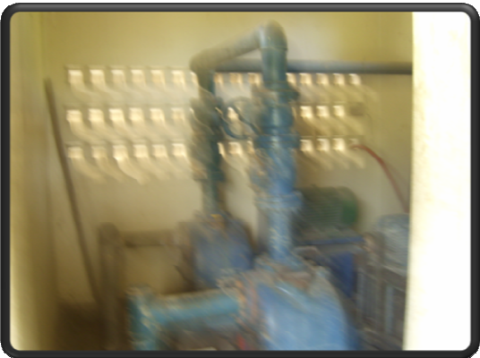
The above picture displays the Piping network and the pumping units at the Glendale Pumping station
