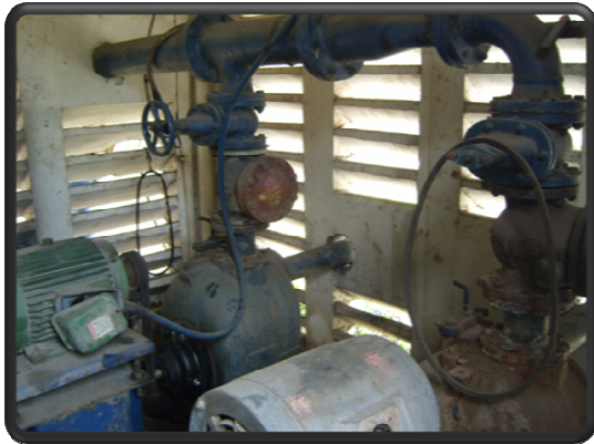
The above picture depicts the general piping network at the Red Hills Rd pumping station
