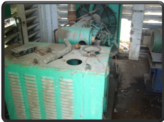
The above picture depicts the general condition of the back up generator inside the building housing them
