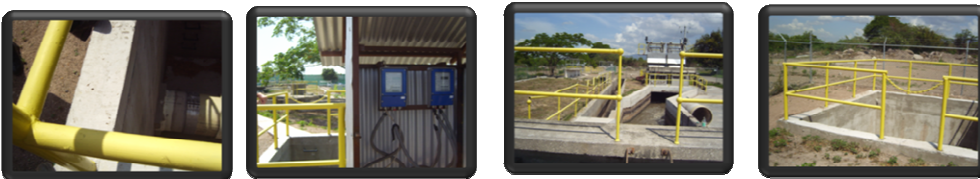
The above pictures display the flow meters and the inlet to the 700mm pipe line used at the Greenwich pumping station
