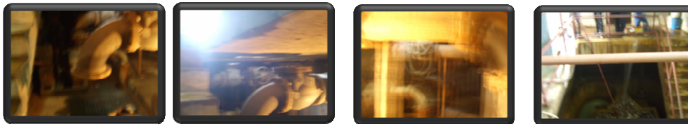
The above pictures display the interior of the lower level of the Seaview Pump
