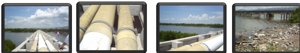
The above pictures display the pipe line that transports the effluent from Nanshe Pen and the Seaview Pumping Station
