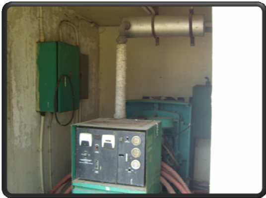
The Above picture displays the back up generator at the facility which is currently out of service
