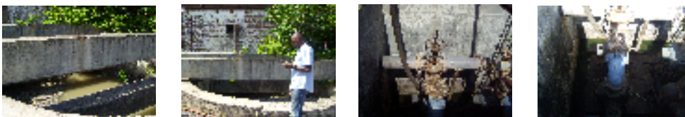
The pumping unit, wet well and the automatic level switch at the Darling St. facility
