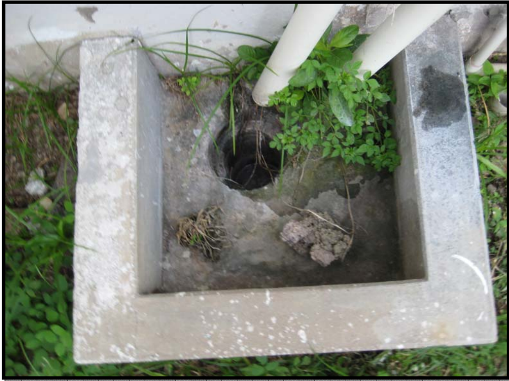
View of Grease trap
