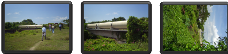
The above pictures depicts the 700mm Fibre glass main line from Greenwich to Seaview Pump Station
