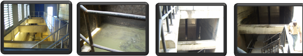
The wet wellll at the facility and the route it take to the outlet point
