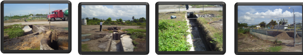
The above picture depicts the inlet point where influent from New port west to the newly installed soapberry channel
