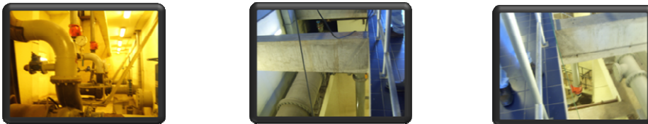
The above images showing the pumps & the 14" outlet pipe which channels to the soapberry
