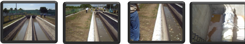
The above picture depicts the water channel installed which leads to the inlet pipes of the soapberry
