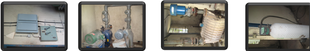
The above pictures displays the electrical panels and controls along with the blower units, pump units and the chlorination unit
