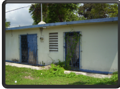
The general overview of the facility at the barbican treatment plant
