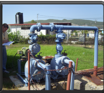
Inlet piping to the pumping unit
