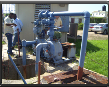
General piping network at the Edge Water pumping station
