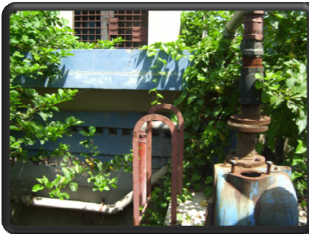
existing pump station at the Christian Pen
