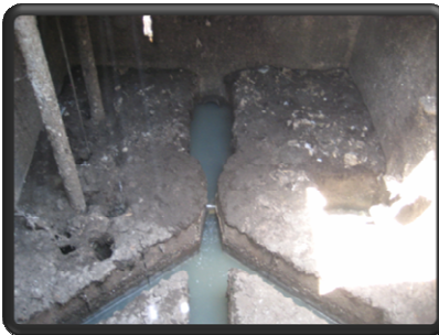
wet well outside and the automatic level switches
