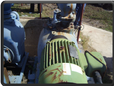
picture depicting the drive motor condition
