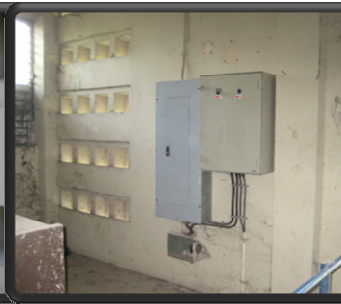
electrical panels inside the
