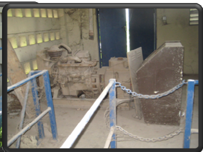
back up generator inside the building
