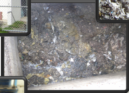
condition of the Wet well at the
