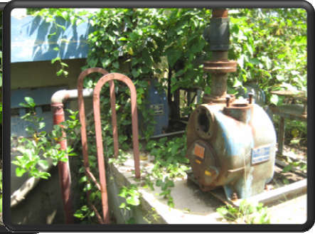
Pictures showing the pump which is currently out of service
