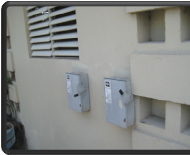
Building housing the electricals and the back up motor
