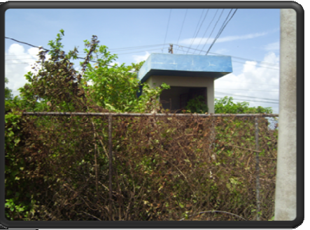
From the main road the general condition of the pumping station covered in vegetation
