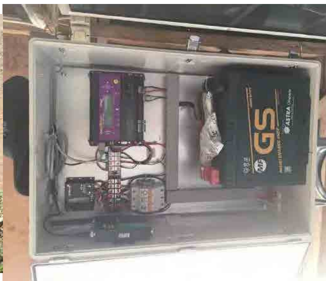
Data Logger and Battery Box
