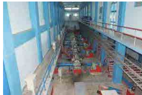
Pomp System at Samba Opu WTP
