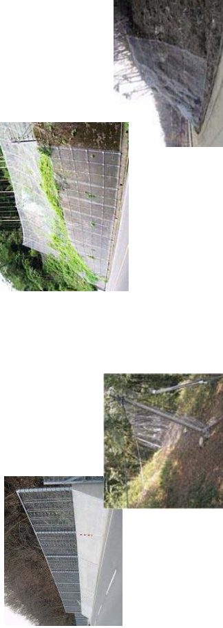
Protection Fence (Japan)
