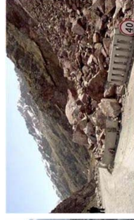
BO Road DEP9
