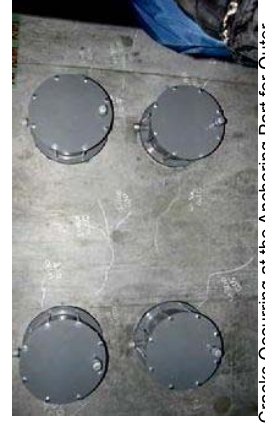
Cracks Occurring at the Anchoring Part for Outer Cables of the Cross Beam
