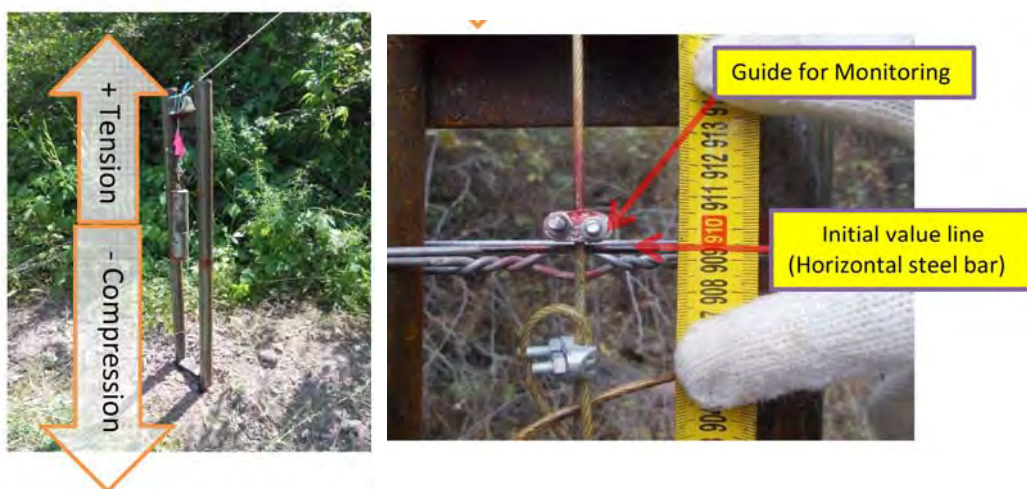
Figure 10-6 Monitoring method at the steel pile and wire type instruments
