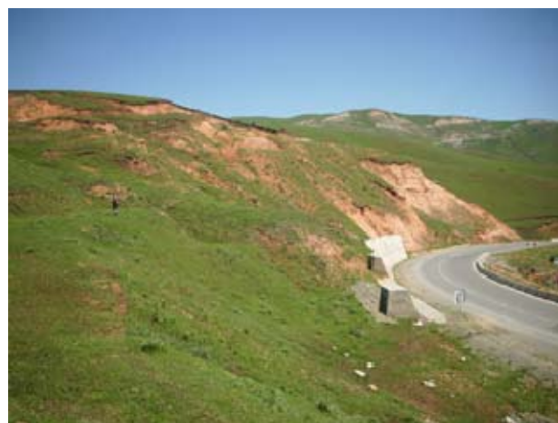
Sliding cliff are occurring due to the moving of landslide (DEP959)
