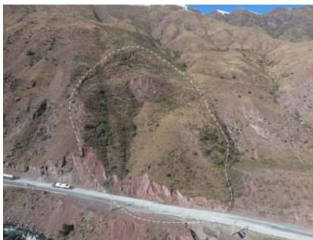
Deformation on the road surface are occurring due to the moving of landslide (DEP9)
