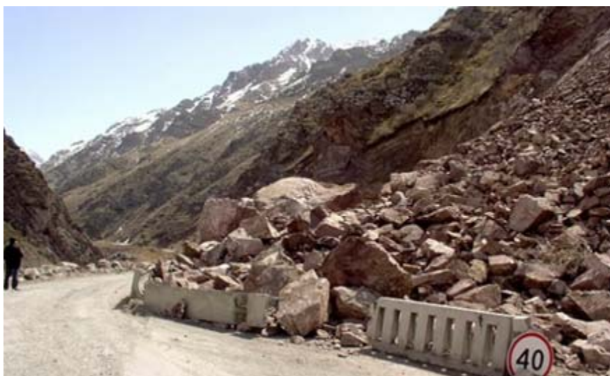
Photo 2.1-2 Accumulated Rockfall at Back of Wall (DEP9)
