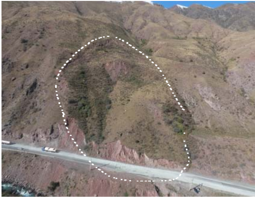
Deformed roadway due to landslide (DEU-9)
