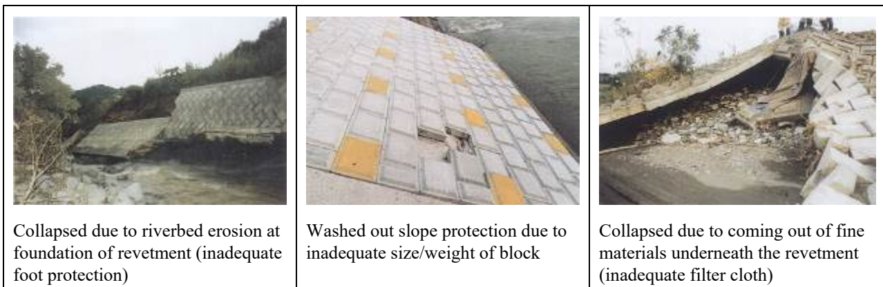
Figure 2.1.4 Sample of Damaged/Collapsed Revetment
