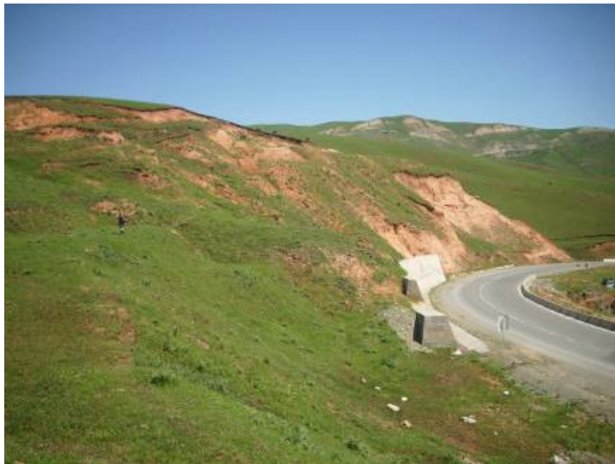
Head cliff due to Landslide (DEU-959)
