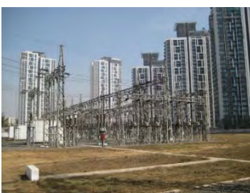
Sector 72 Substation (Gurgaon)
