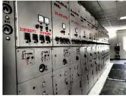
Control panel (Balkampet substation)
