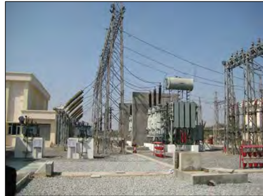
Sector 20 Substation (Gurgaon)
