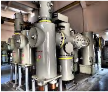
GIS unit (Patigadda substation)
