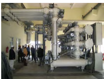
Sector 20 Substation (Gurgaon) Gas Insulated Switchgear (GIS)
