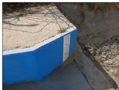
The water flow meter installed by this project
