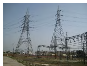
Power Line (Samalhka Substation)
