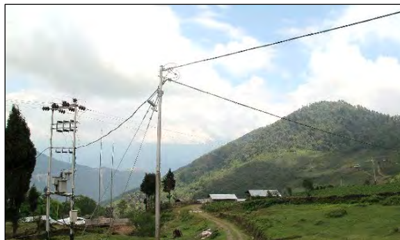
Power Distribution Transformer and 33kV Power Lines (Monggar Dzongkhag, Narang Gewog 2 )
