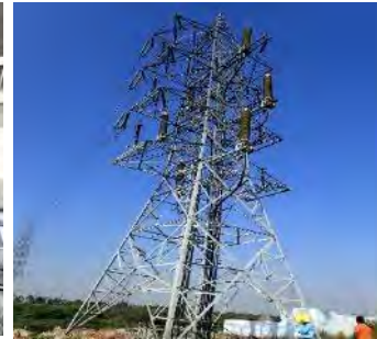
220kV transmission line (between Hayathnagar substation and Ghanapur substation)
