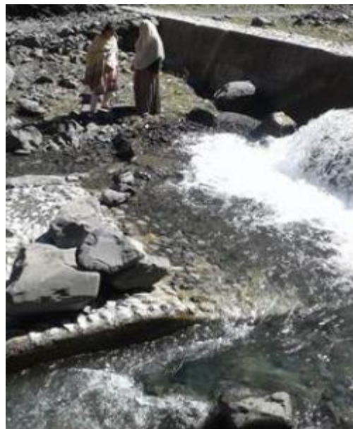
Photo 2. Abundant water flow at Namly Mira water intake facility (taken during interview at site inspection)
