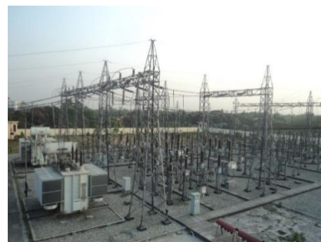
Photo 1. Transformers and transmission facilities (Meghnaghat 132/33 kV substation)
