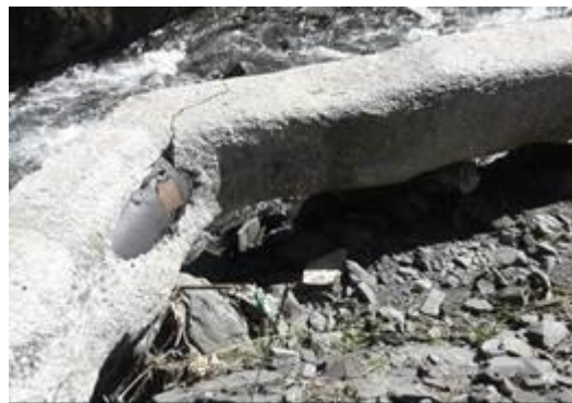
Photo 5. Damage to protective cover of transmission mains at Namly Mira intake facility due to flooding
