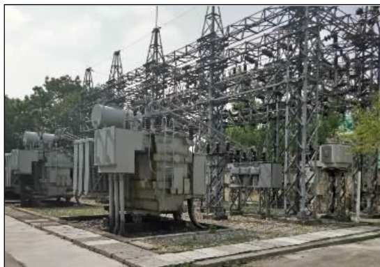
Rehabilitated Substation (Tangail, Sylhet)
