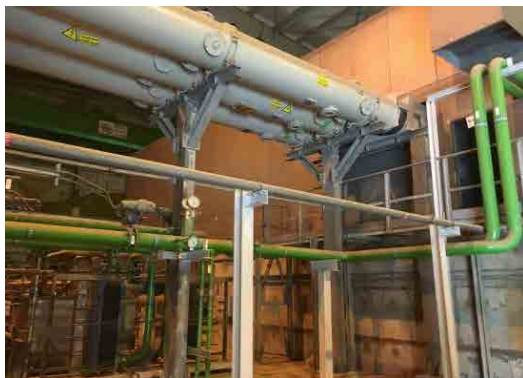
Photo 3: Steam Turbine Room
