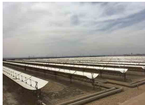
Photo 2: Solar Heat Collectors
