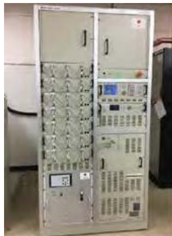
Short-wave transmitter (Henderson Transmitter site)
