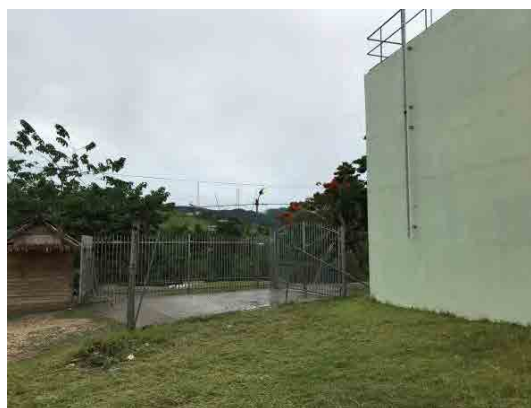
Old fence surrounding the Tasahe pump station where the old reservoir is located
