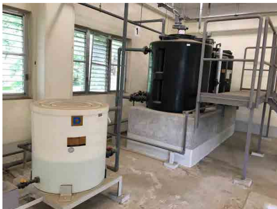
Unused chlorine facility (Tasahe Pump Station)
