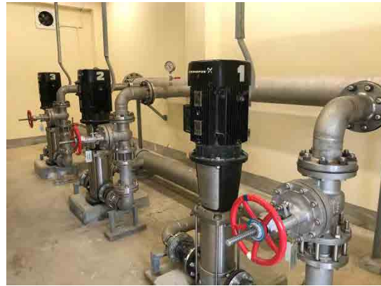
Water Transmission Pump Installed through the Project
