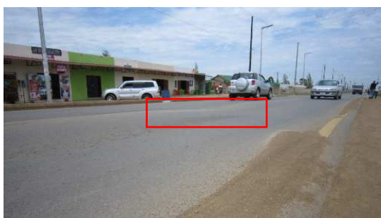
Photo: One of part of road unevenness (The part surrounded by the red frame is sinking)
