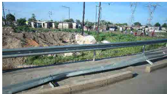
Photo: Damaged guardrails
