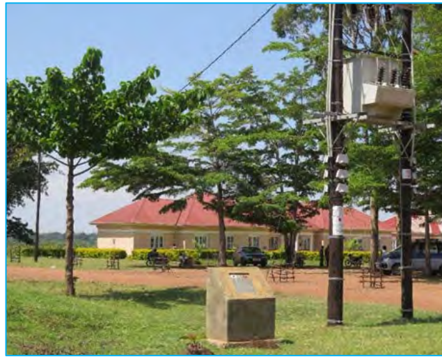
Namayingo District Office electrified by this project and a transformer
