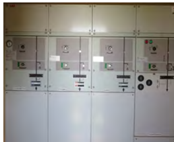
Ring Main Unit (Huye distribution network)
