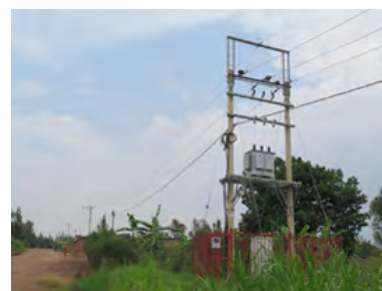
Medium / Low-voltage distribution line joining pole (Kigali City distribution network)
