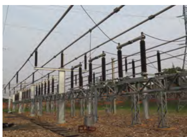
Outdoor switchgear (Gikondo Substation)
