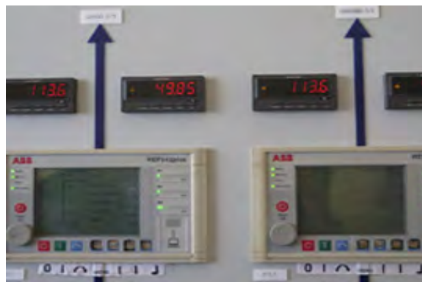
Damaged control buttons of substation control console (Musha Substation)
