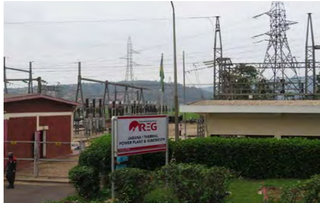
Jabana Substation Refurbished by this project
