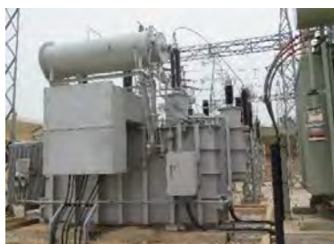
Main Transformer (Musha Substation)
