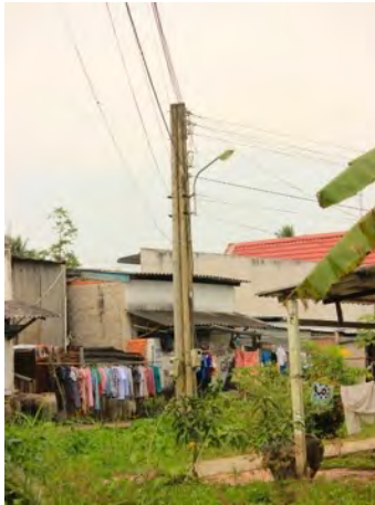
Electricity subproject. Power lines in low-income areas (Soc Trang Province)
