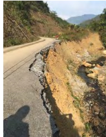
Road subproject. Flood damages (Phu Tho Province)
