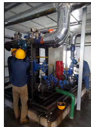
Maintenance of a heat exchange station (Hohhot Chengfa Development & Management Co., Ltd)
