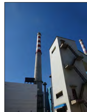
Southeast heat source plant: Chimney for dust collection and desulfurization (Hohhot Chengfa Development & Management Co., Ltd)
