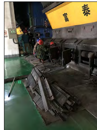
Bayan heat source plant: Boiler maintenance (Hohhot Futai Heating Supply Co., Ltd.)
