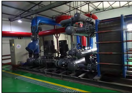
Heat exchange station (Hohhot Futai Heating Supply Co., Ltd.)
