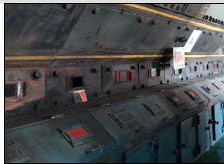
Boiler at Xinjiaying Power Plant B (Hohhot Chengfa Development & Management Co., Ltd)
