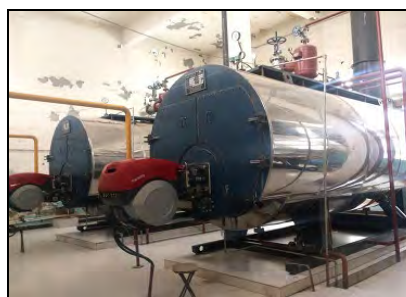
Boiler from the Central Heating Supply (Natural Gas) (Atushi City)
