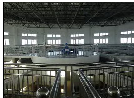
Hami Water Treatment Plant No.4: High-speed Flocculation and Sedimentation Pond
