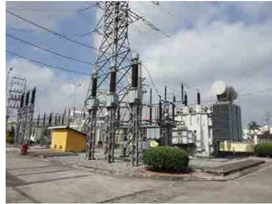
Phuc Dien Substation (Hai Duong Province)
