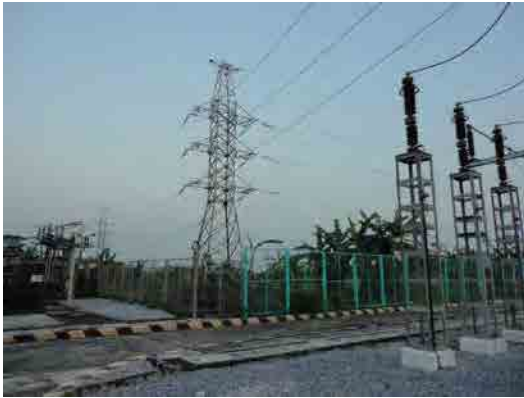
Dong Anh-Chem Transmission Line (Hanoi City)
