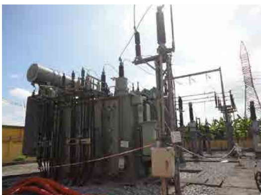
Chau Son Substation (Ha Nam Province)
