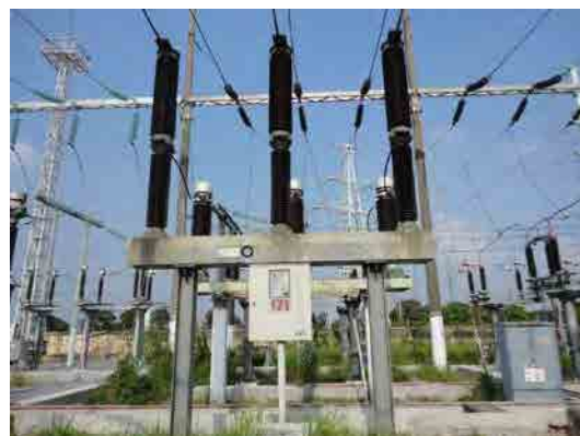
Quang Minh Substation (Hanoi City)
