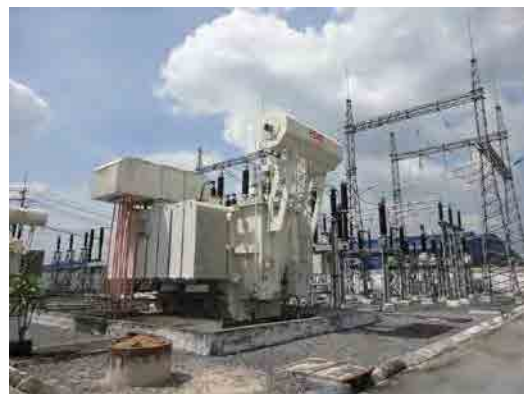
An Phuoc Substation (Dong Nai Province)
