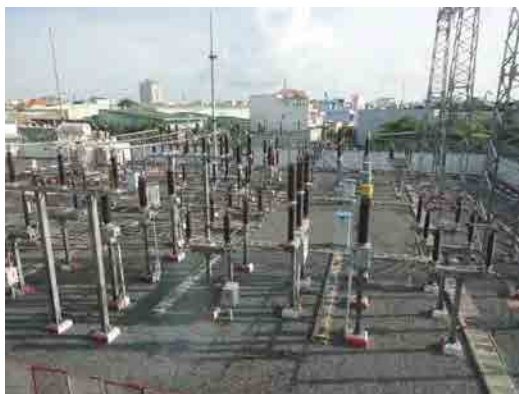
Binh Tri Dong Substation (Ho Chi Minh City)
