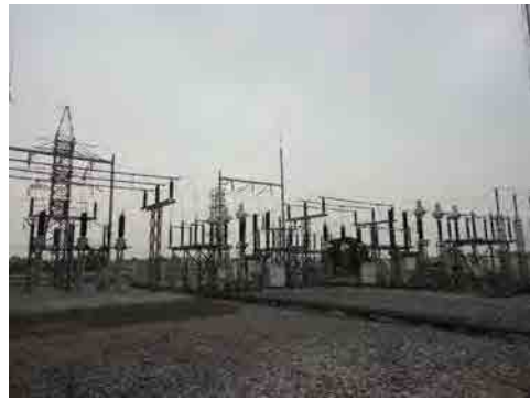
Yen My Substation (Hung Yen Province)
