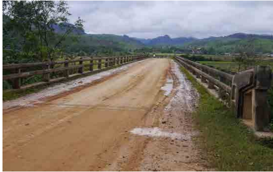
Lac Thien Bridge with dirt accumulation and weeds growing
