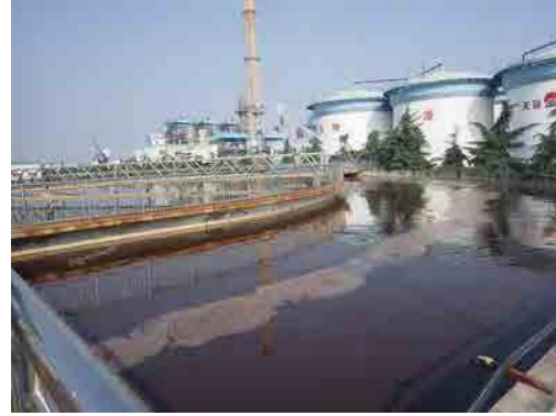
Drainage treatment in the gas production project
