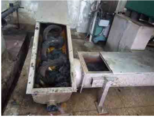
Sludge dewatering process at the North-area Wastewater Treatment Plant
