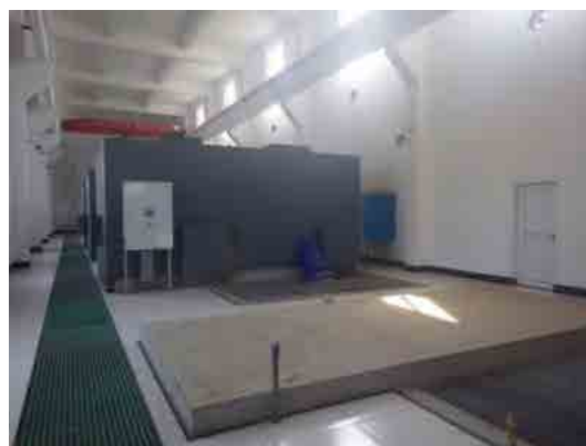
Imported blower at the South-area Wastewater Treatment Plant
