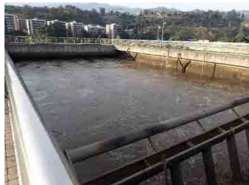
Sewage treatment plant in Panzhihua city
