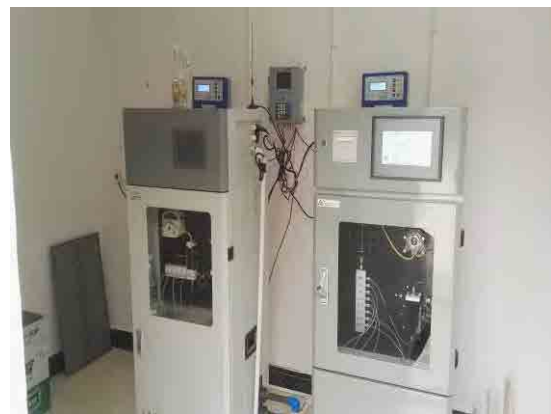
On-line monitoring system for exuded water quality (Sangzhi)
