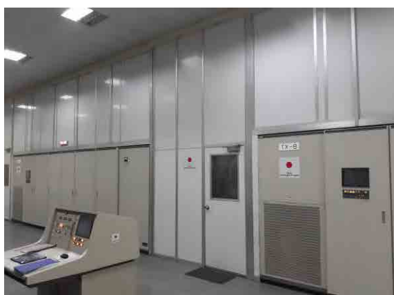
500 kW medium wave transmitter at Faqirabad transmitting station
