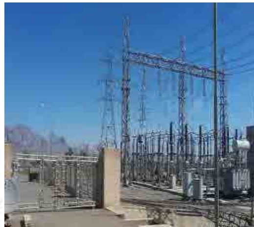
New facility at Khuzdar substation : 220kV powered circuit 3
