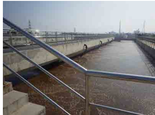
Aeration tank at the South-area Wastewater Treatment Plant (The improved A 2 O process was adopted)
