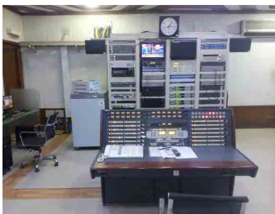
Master control room at the headquarters, Islamabad
