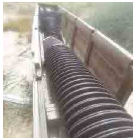
Dadu substation on site 198kV surge arrester(Provided by NTDC)
