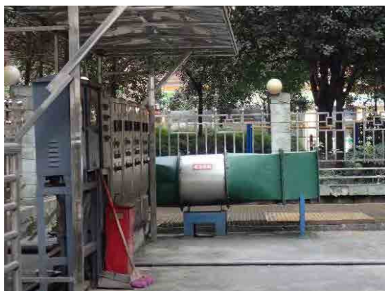
Pump station in Yibin city
