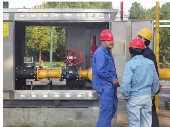
Gas supply regulator station
