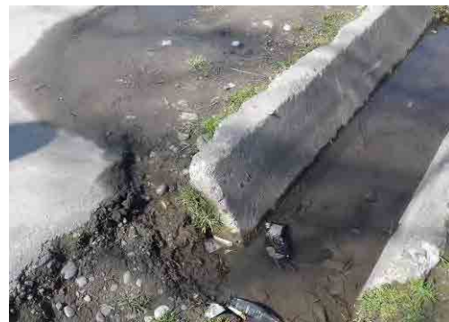
Water Leakage onto Roadways
