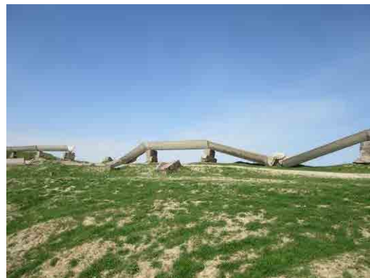
A flume which collapsed after project completion (Qarasha WCA)
