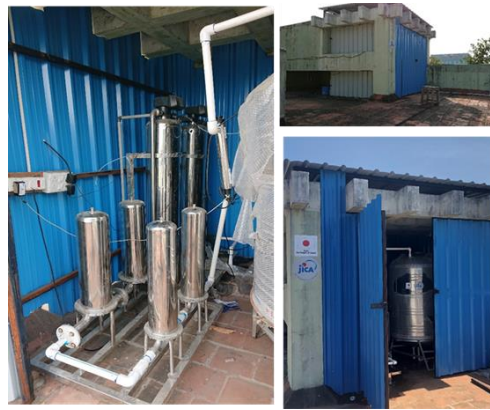
Figure 8 Water Purification Plant installed on the rooftop of SG&SWRDC building
