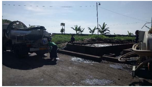
Photo 4.1.3 Septage into C1 WWTP by Vacuum Truck
