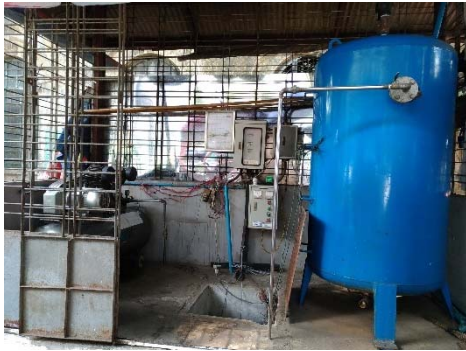
Compressor and Air Tank
