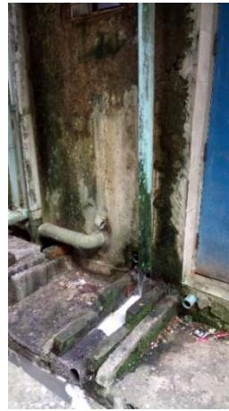
Photo 4.1.5 Existing Drain Pile (Rainwater and Graywater)
