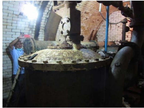
Sewage Tank in Manhole
