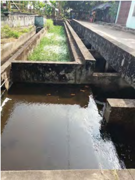
No. 11 Disinfection Tank
