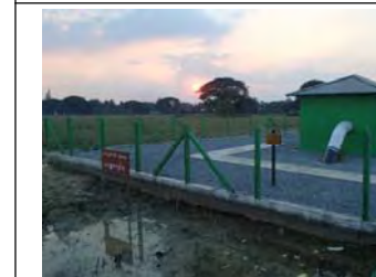
Facility of gas pipeline (North Eastern vicinity of the site)
