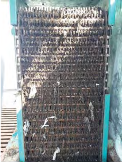
No.2 Auto Bar Screen (Front View)
