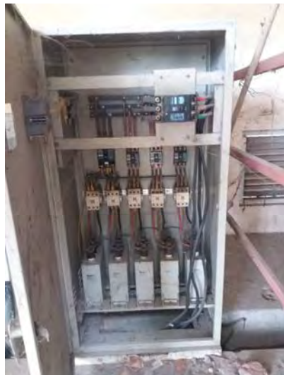
No.2 Capacitor Bank
