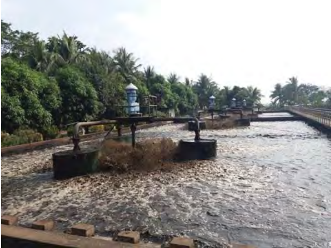
No.8 Aeration Tank (Surface Aerator)
