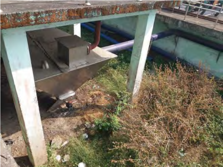
No.5 Grit Separator
