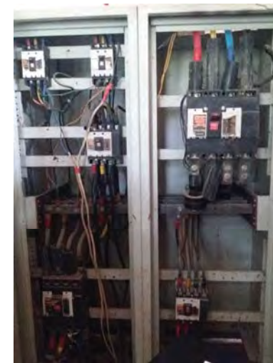
No.4 Distribution Panel (1)
