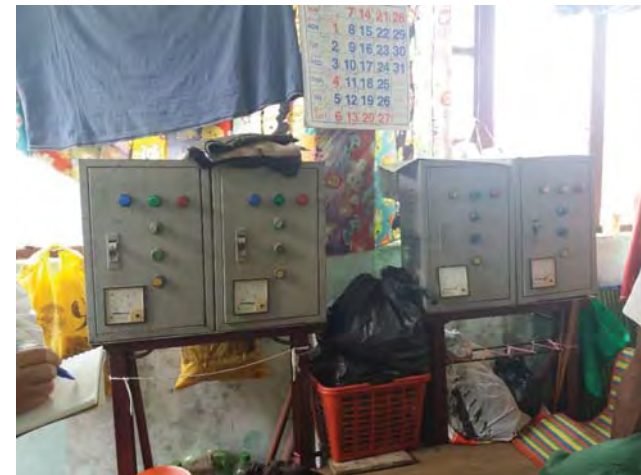
No.7 Secondary Settling Tank Scrapers & Thickener Scrapers
