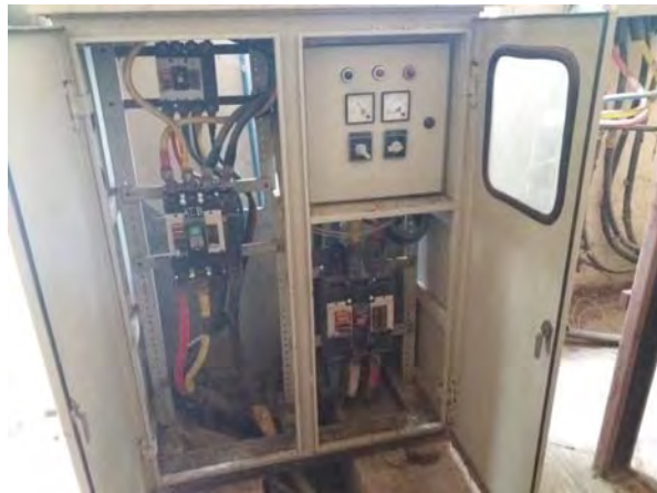
No.5 Distribution Panel (2)
