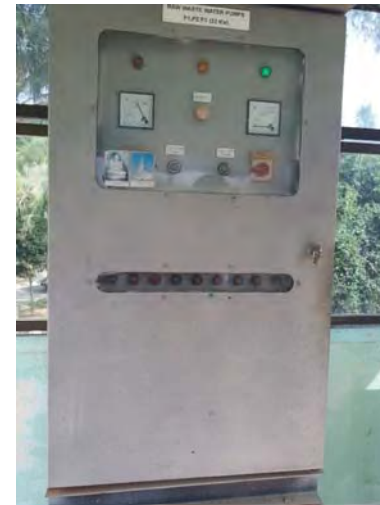
No.11 Raw Waste Water Pump Panel
