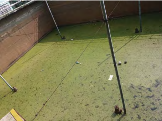
No. 15 Aerobic Digester (Submersible Aerator)
