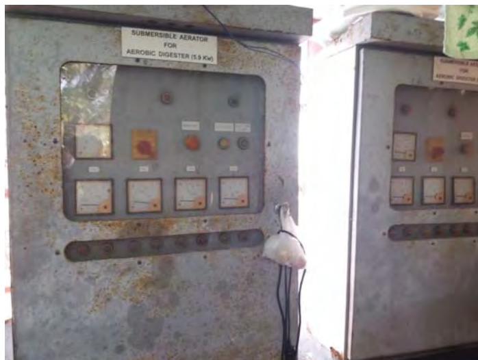
No.6 Aerobic Digester Control Panel
