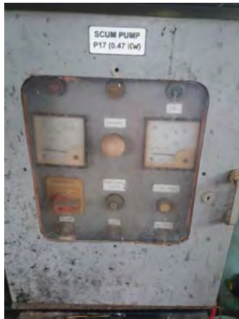
No.9 Scum Pump Panel
