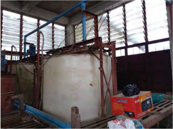
No. 14 Sludge Dewatering Unit (Polymer Dosing Unit)
