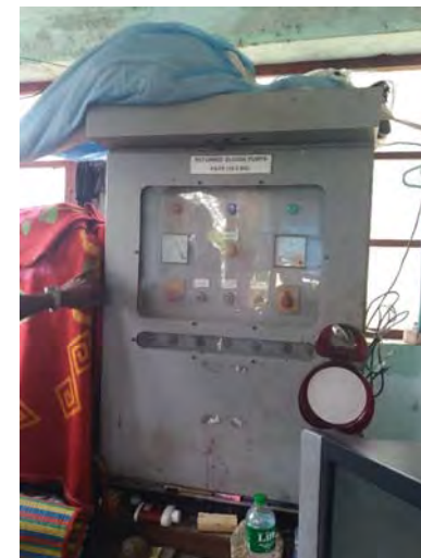
No.8 Return Sludge Pump Panel
