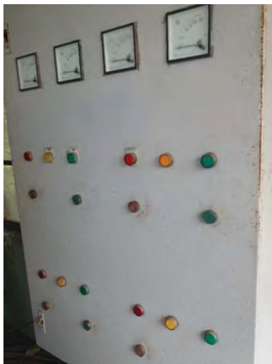
No.10 Surface Aerator Panel
