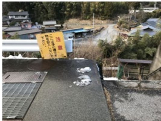
A combined septic tank installed in the village
