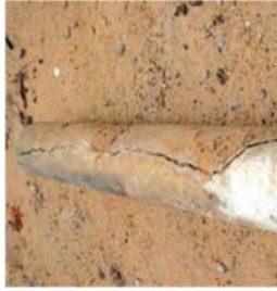
Fig. 6-6 Crack by the water hammer
