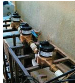
Figure A5-14 Meter Inspection at the Office
