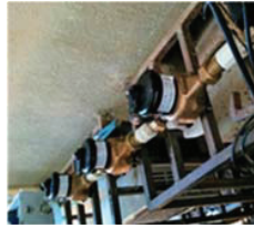
Fig. 2-4 Meter Inspection at the Office
