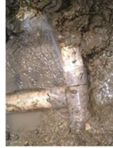
Fig. 6-7 Leak on PVC joint due to less adhesive
