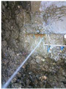
Fig. 6-3 Hole on the galvanized iron pipe
