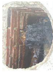
Fig. 4-3 Leak water flow into drain pit
