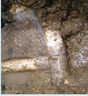
Loose Joint (PVC)
