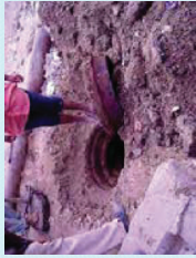
Valve Locating at Site
