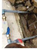
Illegal (Underground Bypassed) Connection
