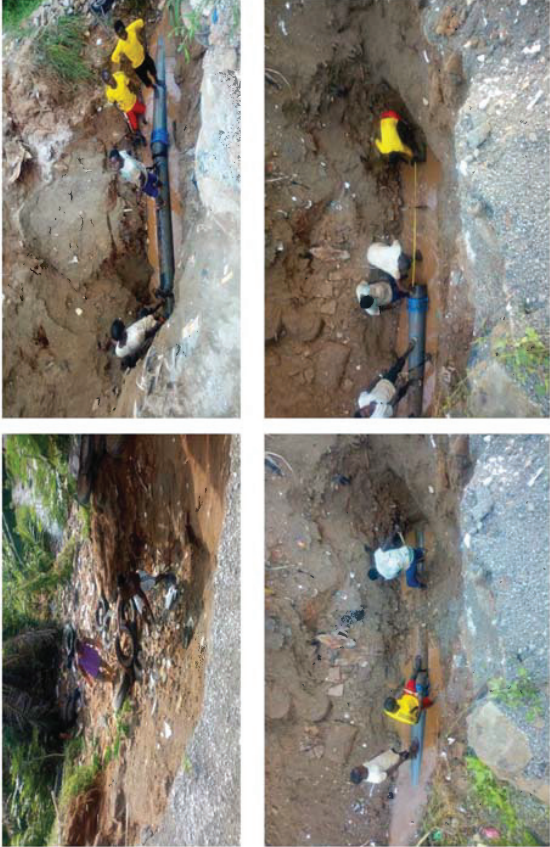
MAINTENANCE OF PIPE BURST
