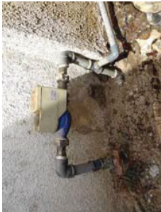
Illegal Bypass in Gudu
