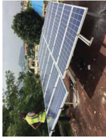
Solar Panels for Zonal Meter
