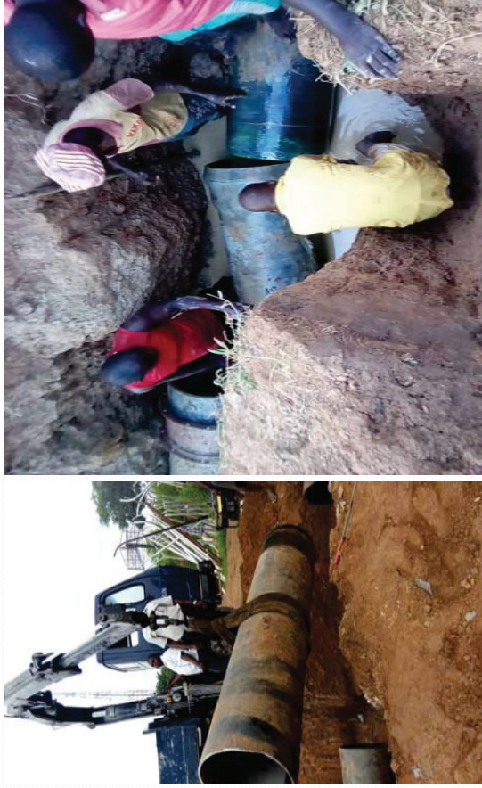
REHABILITATION WORKS ON THE PULL-OUT OF D500MM DUE TO EROSION IMPACT ALONG THE LINE AT NYANYAN AXIS
