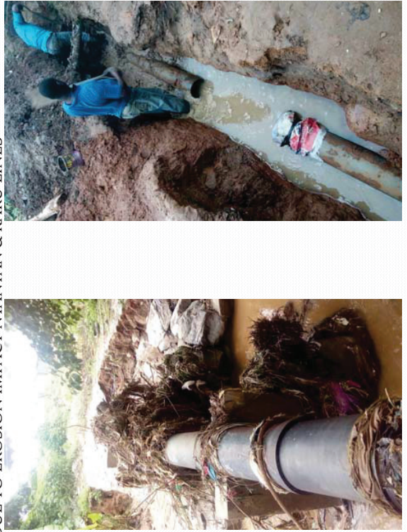
REHABILITATION WORKS ON THE PULL-OUT OF D500MM & 250MM DUE TO EROSION IMPACT NYANYAN & KARU LINES
