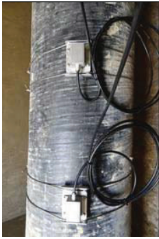
Sensor of Ultrasonic Flow Meter
