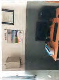
Telemetry System (Monitoring PC)
