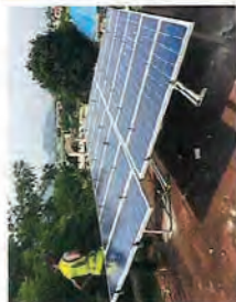
Solar Panels for Zonal Meter
