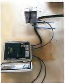
Ultrasonic Flowmeter and Logger for Zonal Meter
