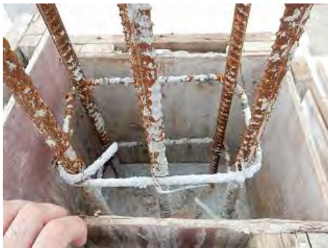
Decentered column rebar
