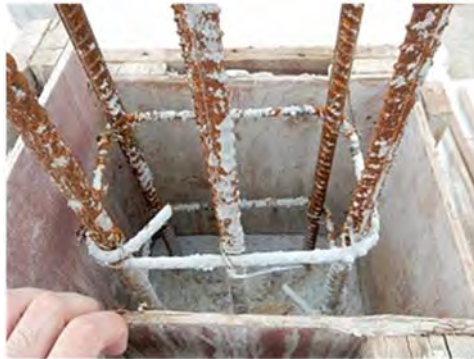
Decentered column rebar
