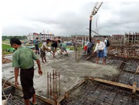
Vibrator inserted askew
