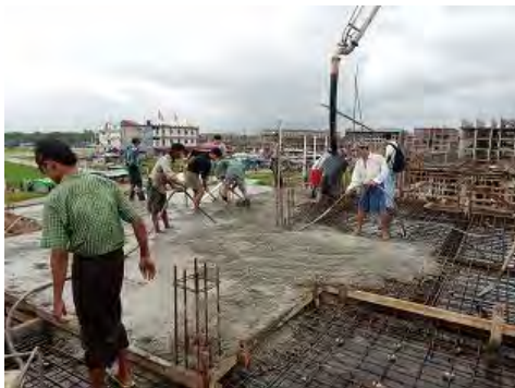
Vibrator inserted askew
