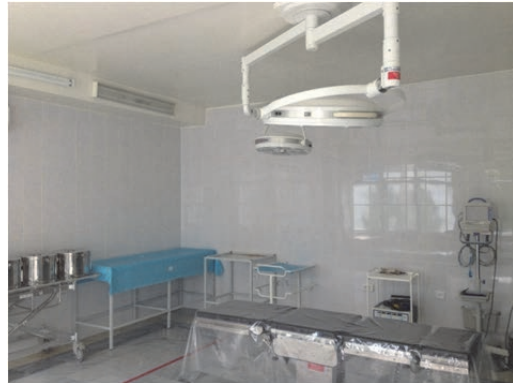
Equipment for Operating Room provide by the Grant Aid Project
