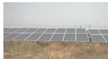
Company C: Solar Power Generation Site
