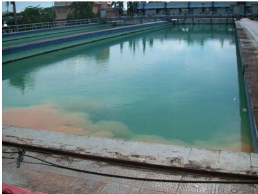
Sedimentation Basin: Raw water is on this side
