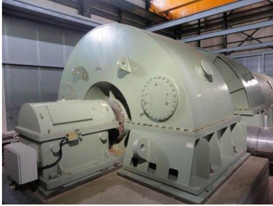
Turbine and Generator
