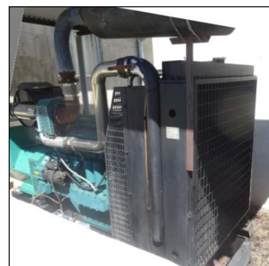
Private power generator at Pilar Water Treatment Plant
