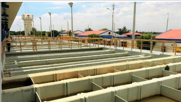
Water Treatment Plant in Piura
