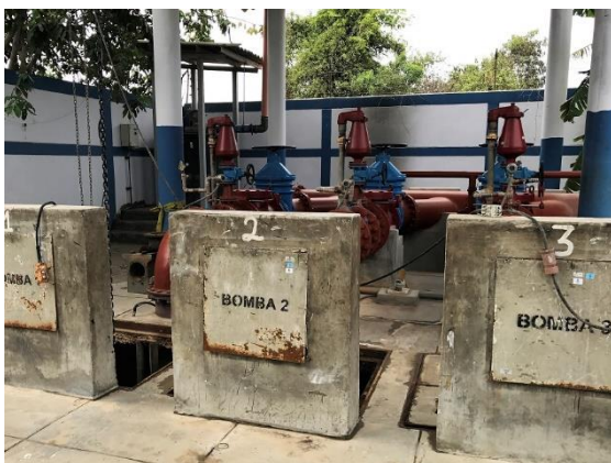
Sewerage pumping station (Piura)
