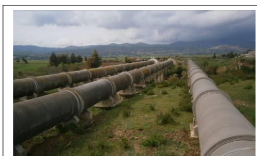
Triplicated Water-supply Pipes (along the Medjerda River)
