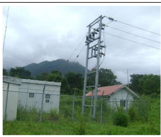
Booster Station and Distribution Line
