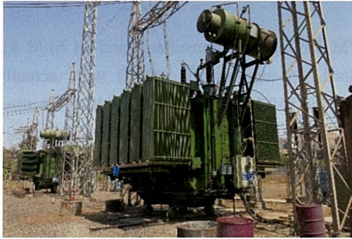
Transformer (Lonawala Substation, Pune Zone)
