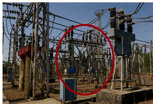
Isolator (Lonawala Substation, Pune Zone)
