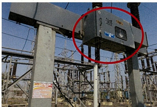
Circuit Breaker (Takali Substation, Nasik Zone)
