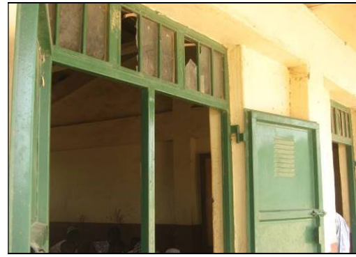
Broken window glass at Tumfafi Primary School
