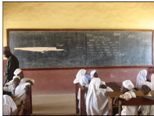
Damaged blackboard at Bichi Kanti Primary School
