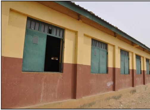
Missing door at Danmadanho Primary School
