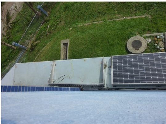
Photo 1: Some solar panels were damaged by typhoon Nock-Ten
