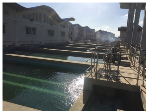
Water Treatment Plant constructed by this project
