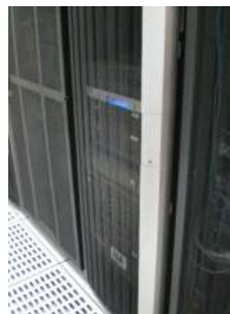
Figure 5 Data management system at EDC headquarters (locked state)
