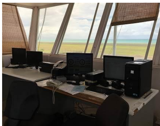
Inside the airport control tower: AWOS Display System (Faleolo International Airport)
