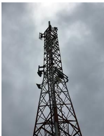
Meteorological Data Communication System (Vaisala)
