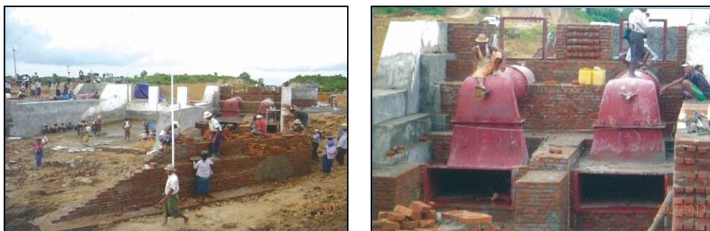
Figure-8 View of Installation of S-shape Tubular Type Power Generation Units (20 kW)
