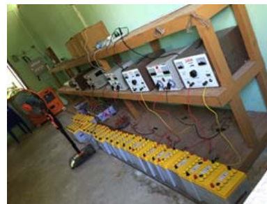
Battery Recharging System
