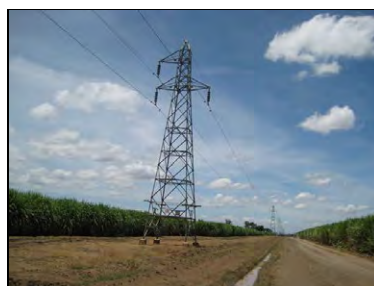
66kV Transmission Line
