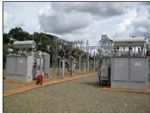
Makuyuni Substation newly installed by the project
