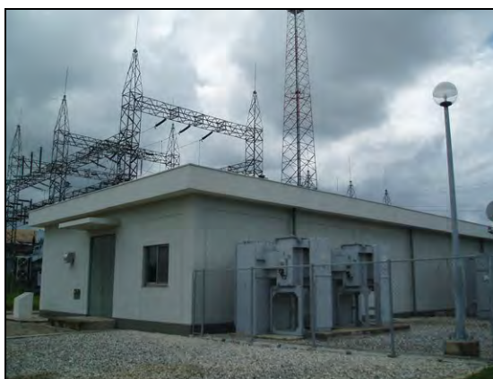
Mtoni Substation expanded by the project (33kV) (adjacent to the 132/33kV Substation that was constructed by the MCA-T Project)
