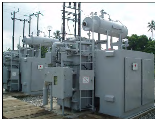
The main transformer of Welezo Substation (33/11kV) newly installed by the project
