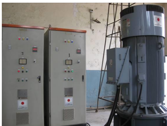
Motor and Electrical Control Panels (Multan Road Pumping Station)
