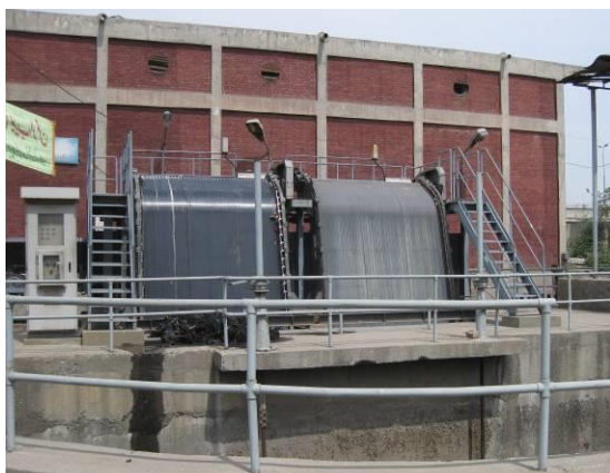
Automatic Trash Rake System (Shad Bagh Pumping Station)
