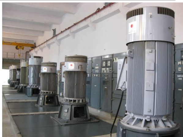
Operation and Electric Room (Gulshan-E-Ravi Pumping Station)
